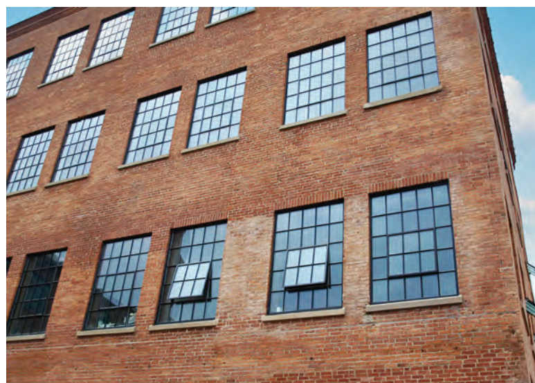
Cable Mills — Williamstown, MA • Reengineered a window with a floating vent that achieved approval from the National Park Service
